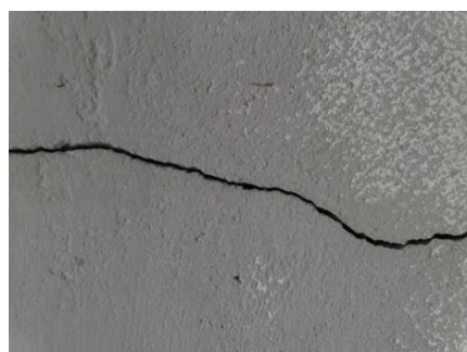
Figure 20: Test Crack 2 Picture
